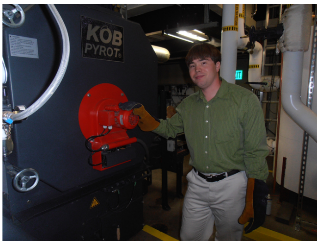
Fig. 2. Nathan Soboleff, a young Tlingit business leader, displaying Sealaska Corporation’s wood-pellet based boiler, which has significantly lowered the firm’s heating costs and carbon emissions.
